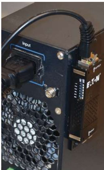
Eaton EMP Gen 2 installed on UPS
